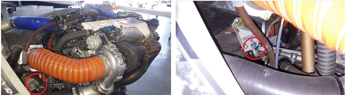
Figure1 - Left: general location of bonding cable at right rear of engine. Right: zoomed view.
