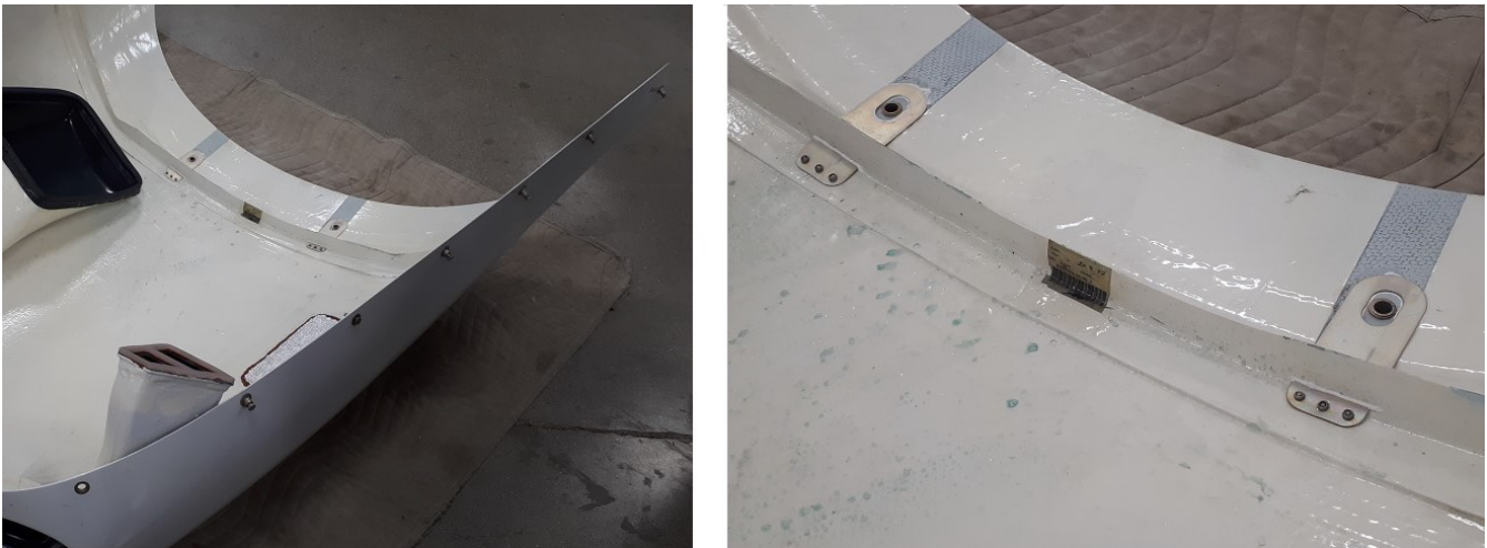
Figure 3. Left: installation of item 2 (x2) on the top cowling. Right: zoomed view. Not shown: apply Nycote to the rivet shanks on the inside of the cowling after the sealant has cured (step 38).
